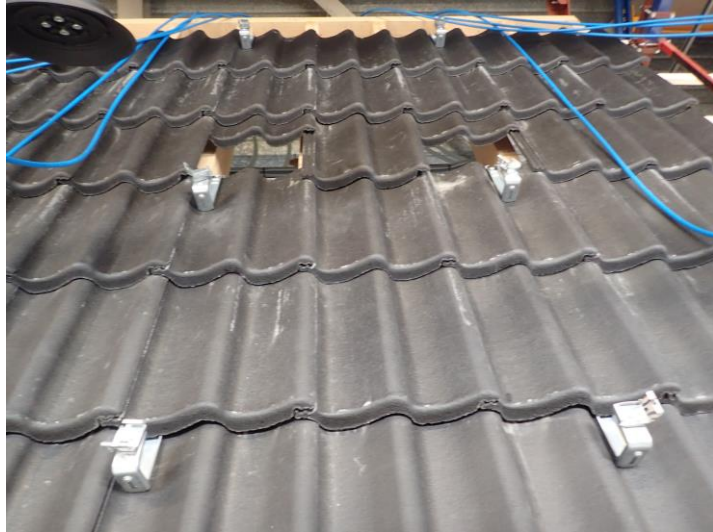
Photo 13 Overview of the system with the roof hooks placed in position for a test on PV-modules in landscape layout.
