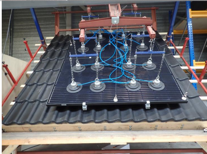
Photo 17 Two PV-modules have been placed on the mounting rail and have been fastened. Also the suction cups are positioned.
