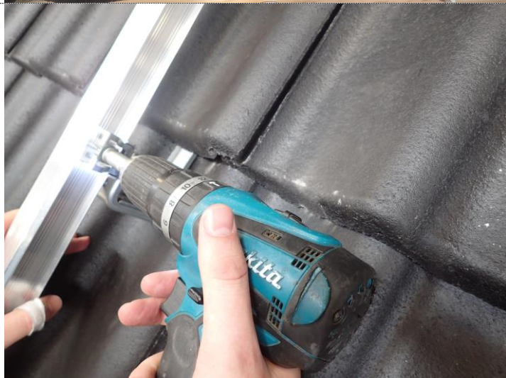
Photo 15 The mounting rail is locked with a screw to the lower roof hook.
