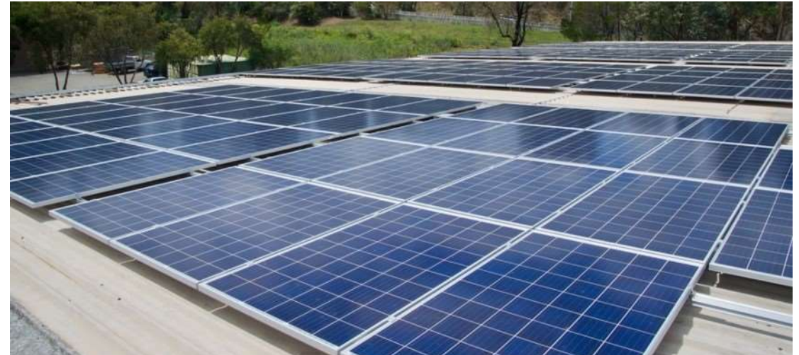
Achieve Energy Solutions
