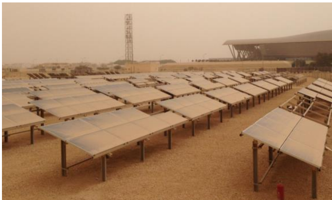
Figure 1: Soiled PV modules, image was taken at the STF of QEERI after a dust storm in Doha, Qatar.
