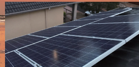
3.6KW | Melbourne, Australia
