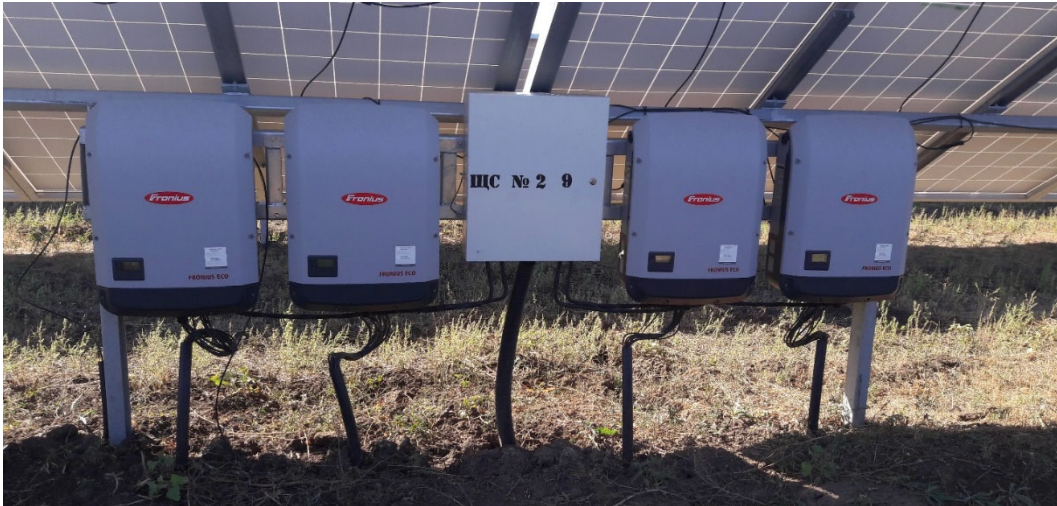
Figure 10: Example showing the groups of 4 inverters - Tokmak system (photo credit: Fronius)
