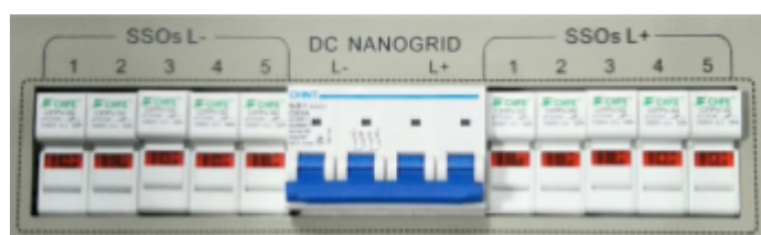
DC Distribution 5 - A02
