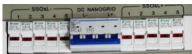
DC Distribution 15 - A02
