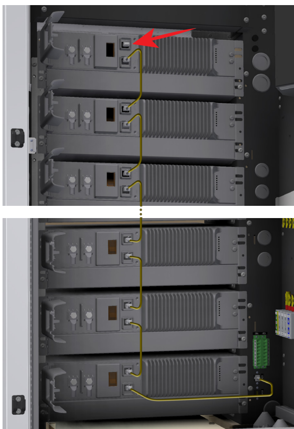
Figure 4.36 Battery communication cables
