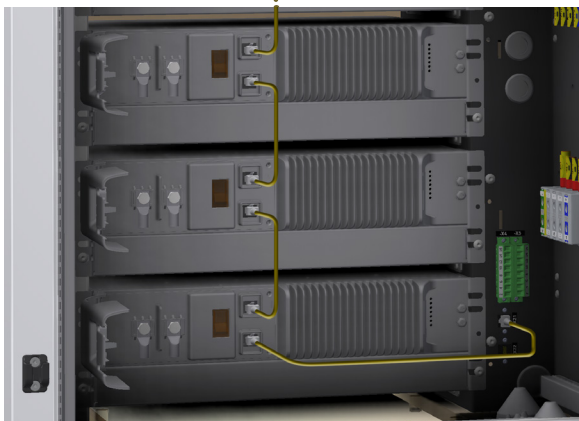
Figure 4.26 Battery communication cables
